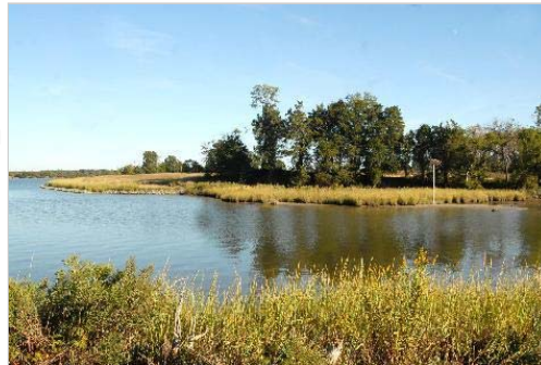
The shoreline restoration project at the Wye House property took four months to complete.
